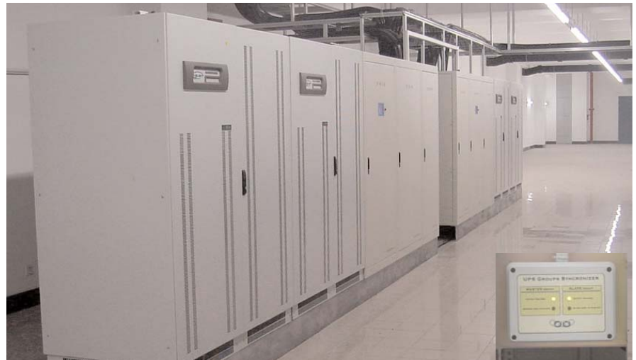
One of the parallel 250kVA Master Dialog UPS Systems and the USG accessory
